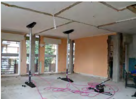
Push load test on a ceiling using COD25N260 cylinder during extraordinary maintenance works in a residential building. Milan, Italy.
