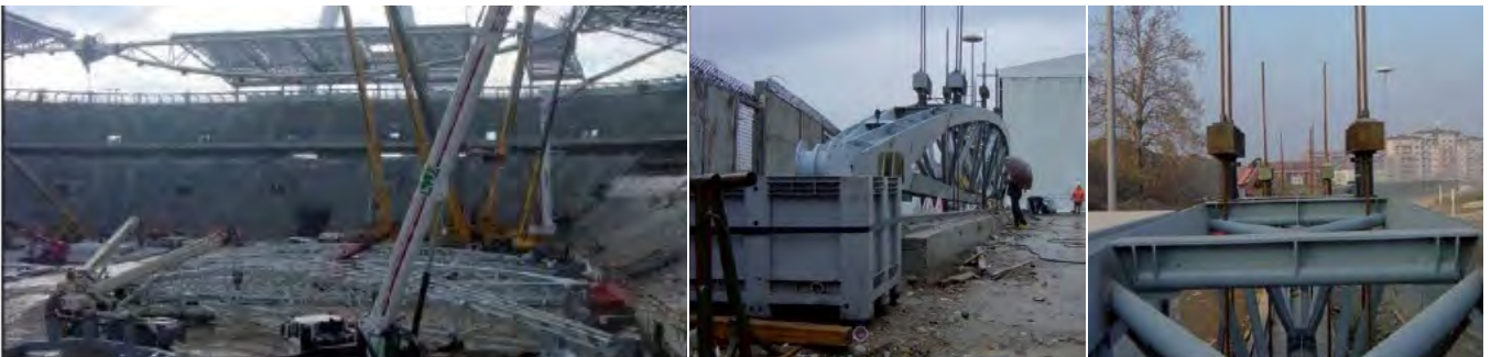
Beams tensioning of the roof of the new Juventus Stadium. Turin, Italy.
